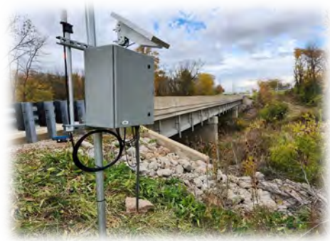
Example of Monitoring Station Equipment
